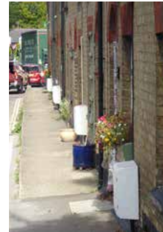
Figure 91: Meter boxes on Kingsland Terrace
